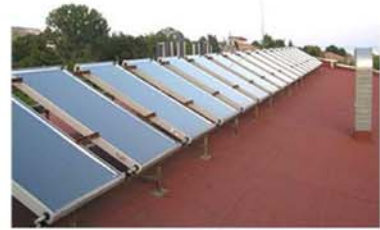
Balchik, Bulgaria, solar collectors on the roof of a hotel
